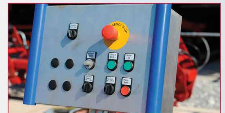
Emergency stop buttons, located in the cabin and on all machinery, are readily available to halt an operation should an unsafe condition occur.
