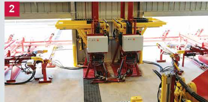
2 Each pipe is lifted onto a walking table and moved to the automated thread-protector remover. The thread protector is removed from one end of each pipe.
