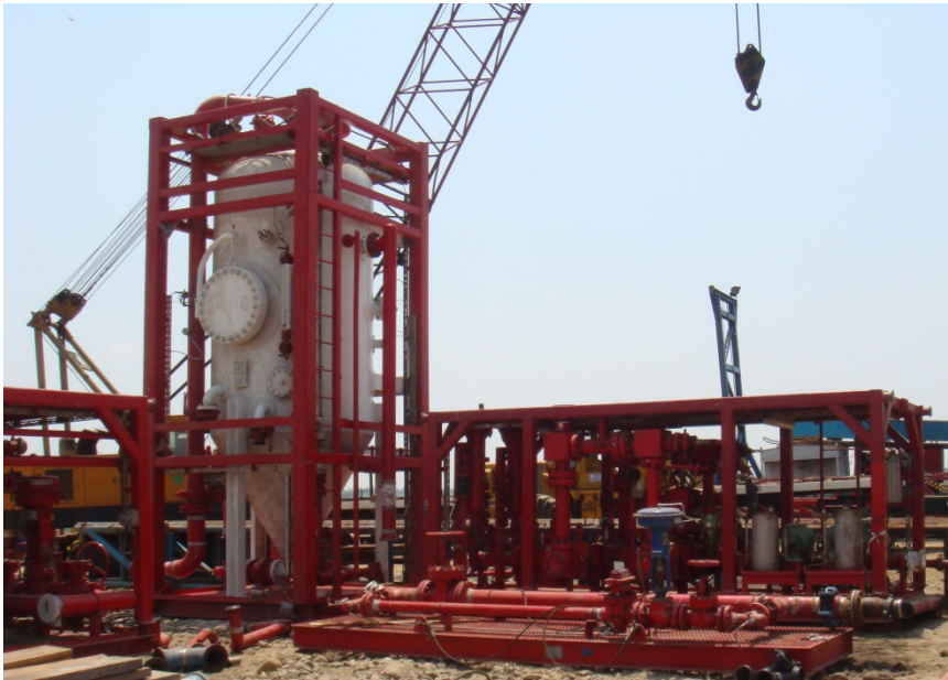
Weatherford provided the full UBD package, including UBD choke manifold, four-phase separator, emergency shutdown, 120-ft (37-m) flare stack, and data-acquisition system.
