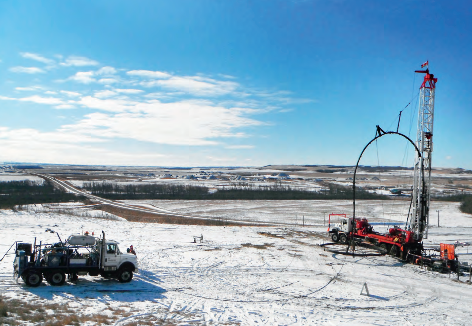
Weatherford COROD® continuous rod deployment in a heavy oil well, Northeastern Alberta.
