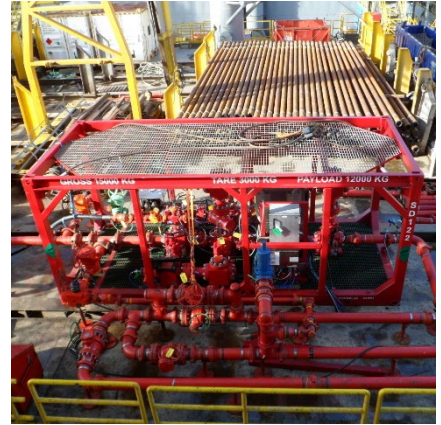
Managed pressure drilling and cementing equipment required only a small footprint for installation.
